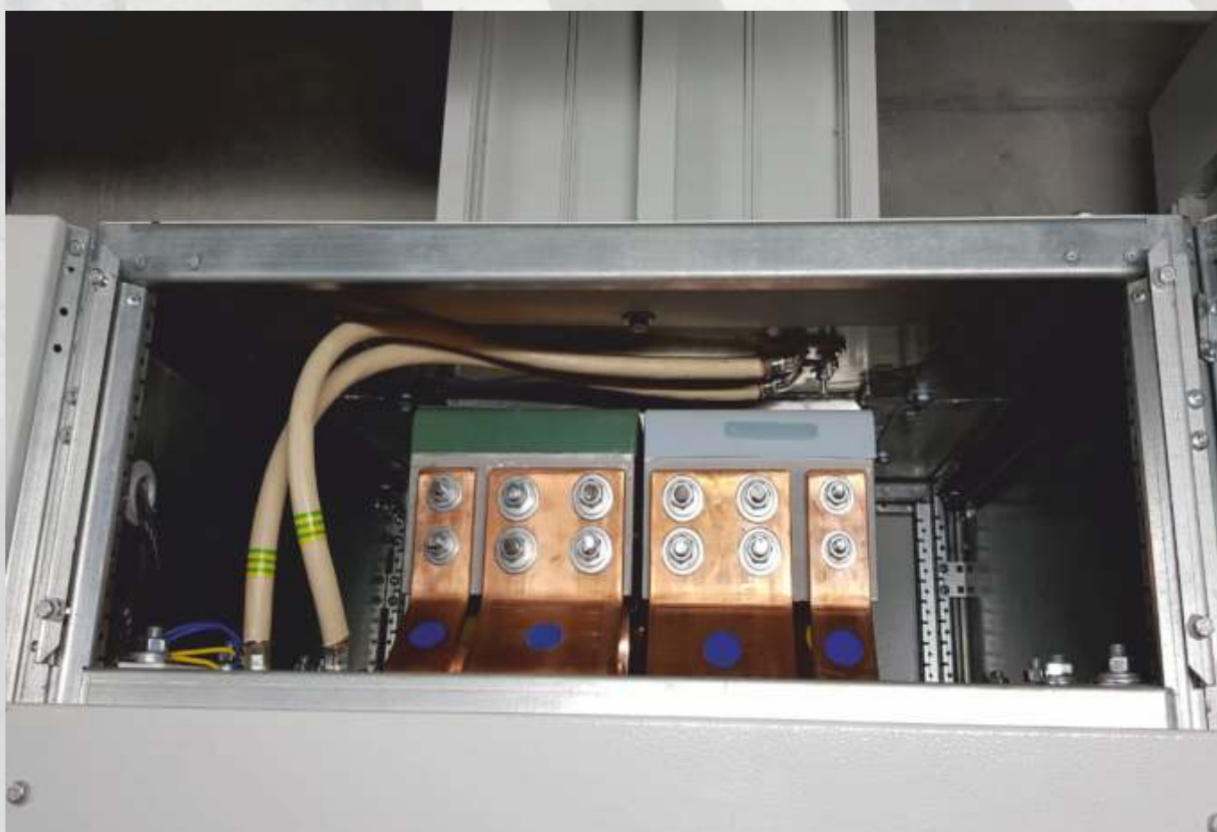
COSMOS shopping mall, Chelyabinsk 2500A busway
